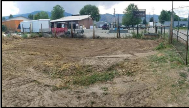
Above: Before and after of the clean up of the Minnie Street entrance of the Salmon School Garden. THANK YOU to Greg Roach Grading and Excavation for donating his time and equipment to tidy up this area!
